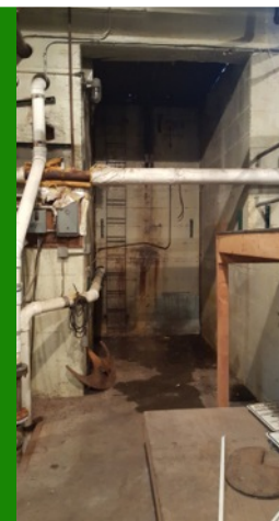
Address moisture issues
